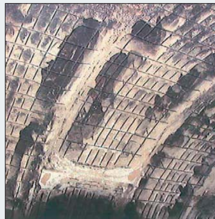
Picture 2 - Lining loss of thickness vary according to reinforcement density
